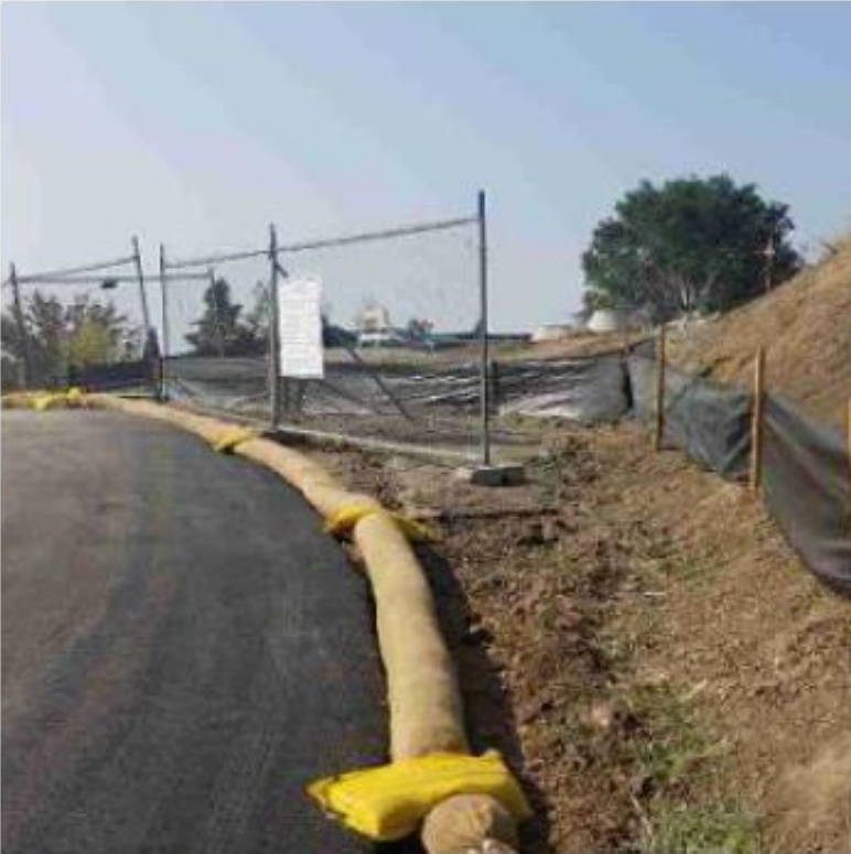
Silt fence has been added and streets were swept.
