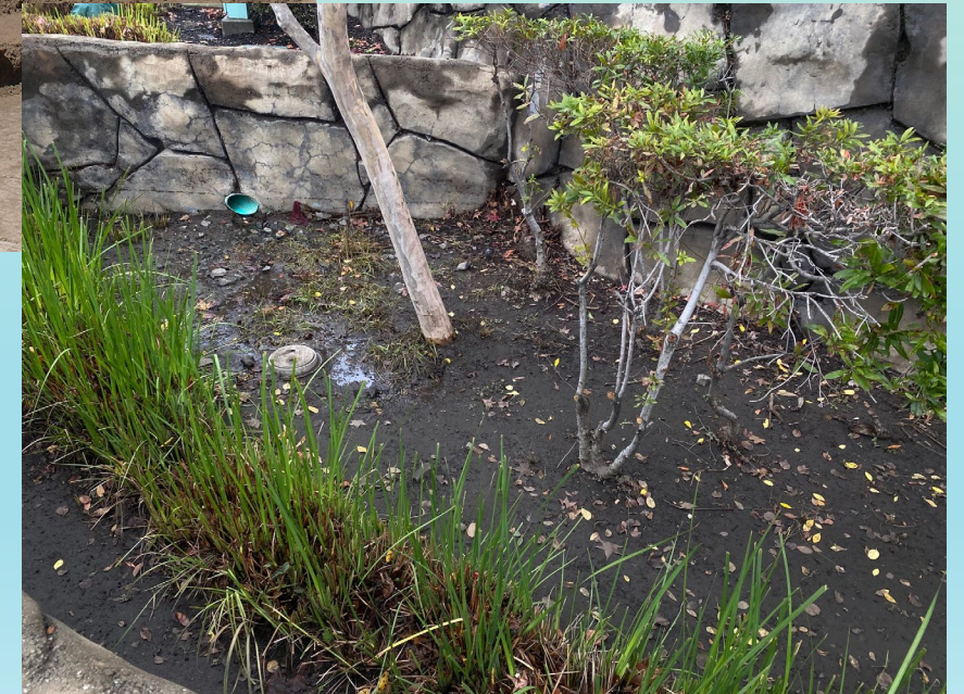
Belmont Terrace Swales flooding due to erosion and sedimentation from surrounding slopes - 2023
