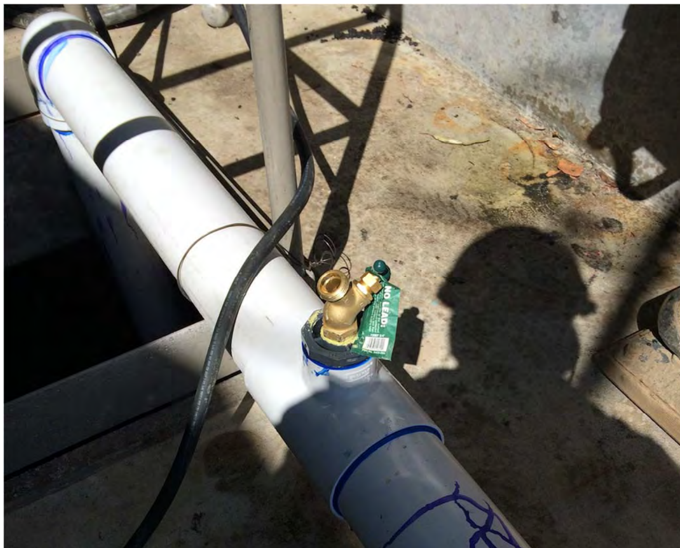
Figure 1. Monitoring Spigot at Diversion Pipe
