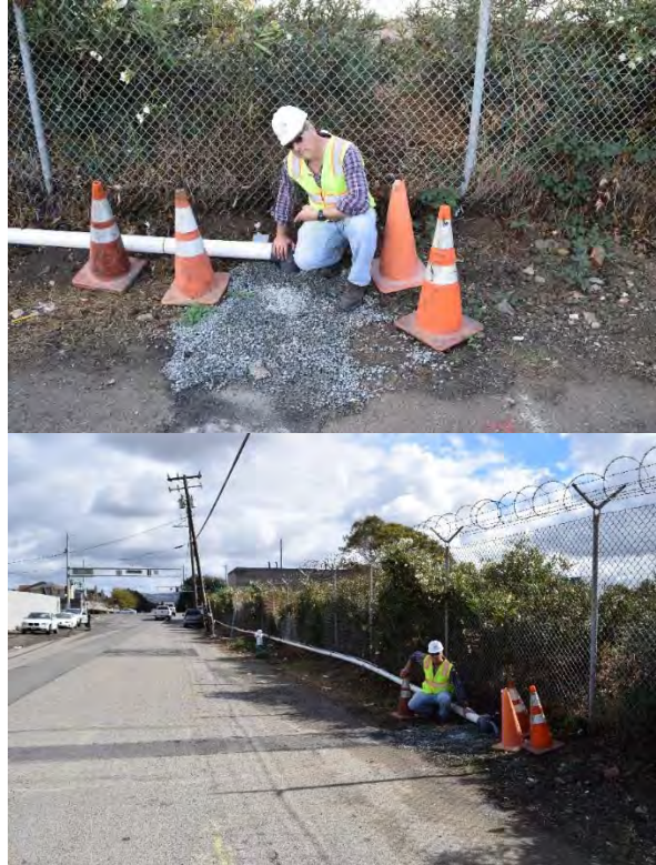
Figure 5 Permanent Manhole Connection to WCWD Linked to the NRSPS via a Temporary Pipe Aligned Along West Gertrude Avenue
