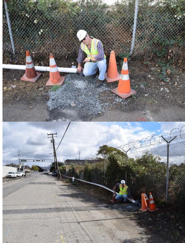
Figure 5 Permanent Manhole Connection to WCWD Linked to the NRSPS via a Temporary Pipe Aligned Along West Gertrude Avenue
