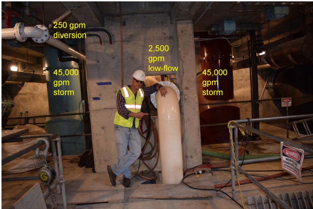
Figure 6 Comparison of the Pipe Sizes Conveying 250 gpm Diversion Flow, 2,500 gpm Low Flows, and 35,000 gpm storm flows
