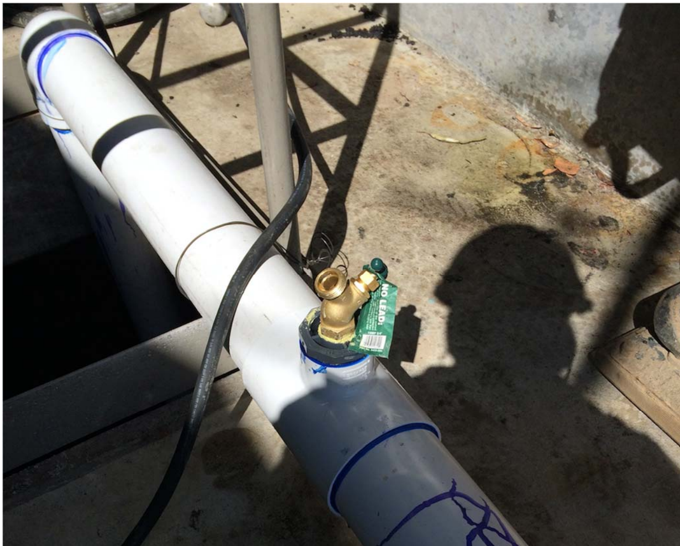
Figure 1. Monitoring Spigot at Diversion Pipe
