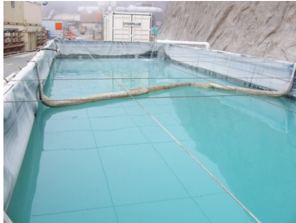
Figure C-3. Sedimentation Tank (Devil's Slide)
