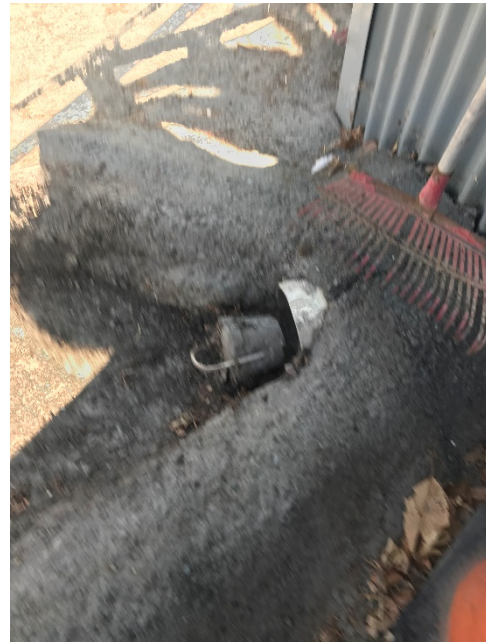
Photograph of dump station to wash pad drain plug
