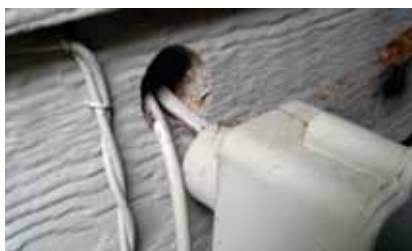
Hole and gap in a wall that will allow insects and rodents to move into, out of, and around a building
