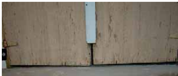
Gaps under and between double doors through which rodents and insects can easily pass
