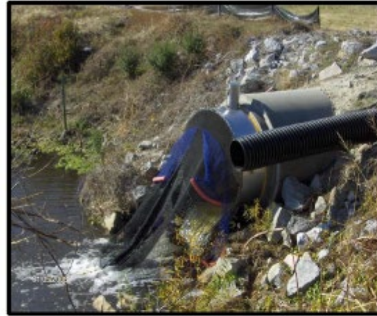
Figure 1. 72" RCP at continuous flow installation.
