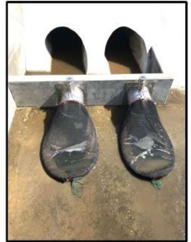
Figure 5. Installed NetTech at approximately 50% capacity.
