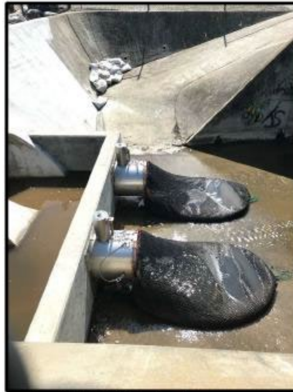
Figure 4. Installed NetTech with maintenance access road.
