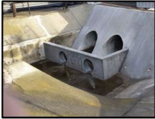
Figure 2. Unusual outlet size and shape.
