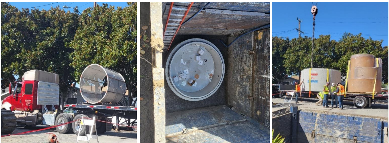
Figure 3.2. Contech CDS® hydrodynamic separator installation in City of Hayward (Image courtesy of EOA, Inc.).
