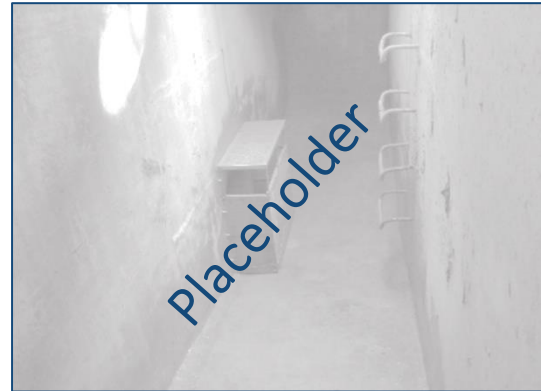
Figure 3.10. Very large HDS unit in San Jose that requires confined space entry to maintain (Image courtesy of City of San Jose staff).
