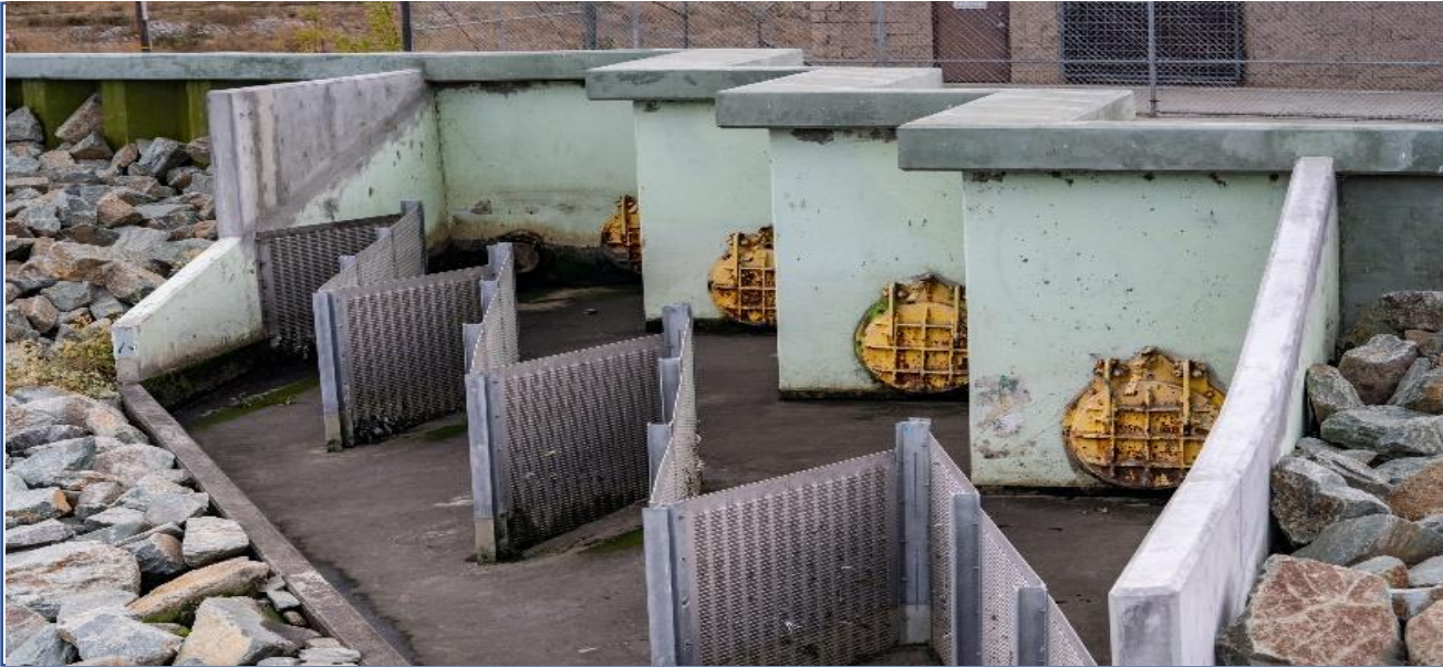
Figure 3.5. Roscoe Moss Gross Solids Removal Device (GSRD) inclined screen configuration installed in the City of East Palo Alto at the outlet of a pump station (Image courtesy of Schaaf and Wheeler Consulting Engineers).
