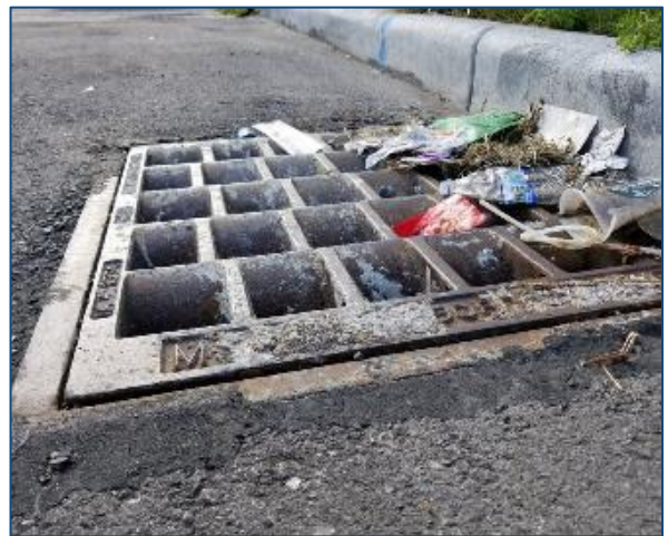
Figure 1.1. Trash accumulating on a storm drain inlet (Photo courtesy of the Santa Clara Valley Urban Runoff Pollution Prevention Program)
