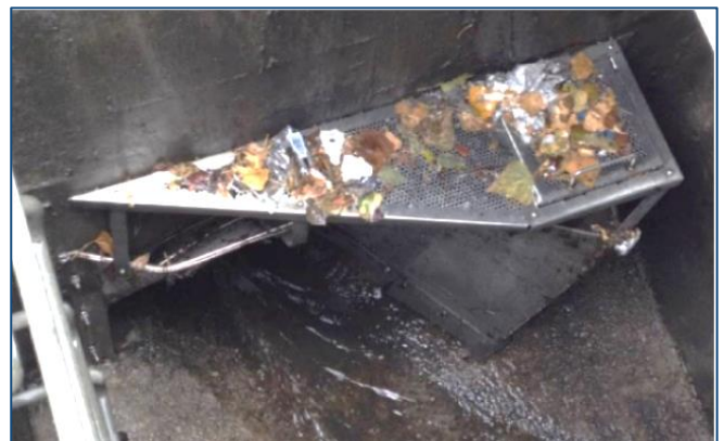
Figure 4.8. Damaged (collapsed) outflow screen type of FTC device (Image courtesy of SCVURPPP and SMCWPPP - EOA)
