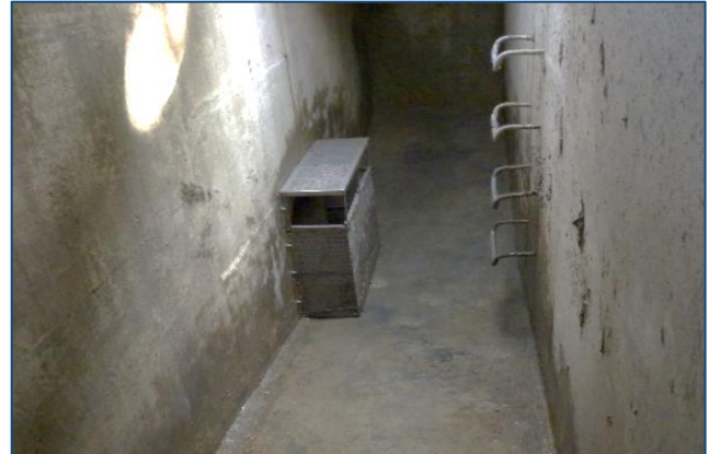
Figure 4.7. Outflow screen installed in a catch basin that requires confined space entry to maintain ( http://unitedstormwater.com/cps.php ).
