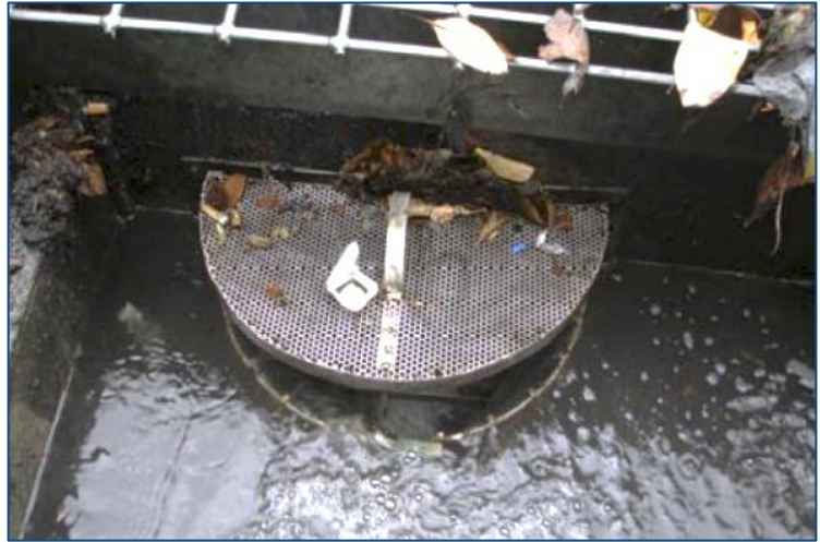
Figure 4.6. Overflowing outflow screen FTC device due to a clogged/occluded screen. Courtesy of SCVURPPP and SMCWPPP (EOA 2016).
