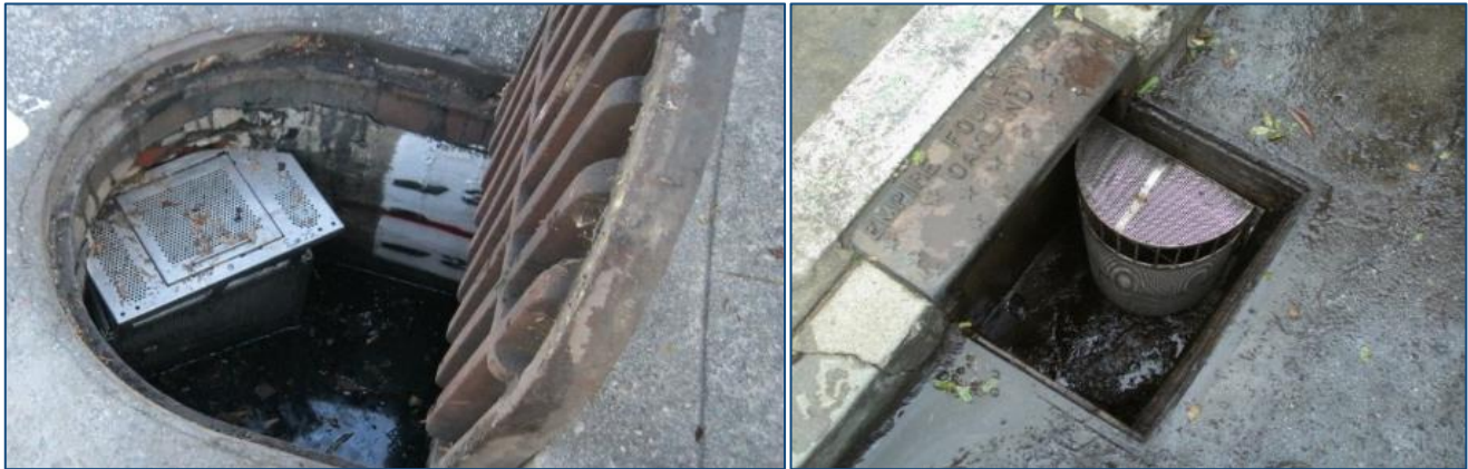
Figure 4.1. Outflow screens installed in catch basins within the Bay Area (Image courtesy of EOA, Inc.).
