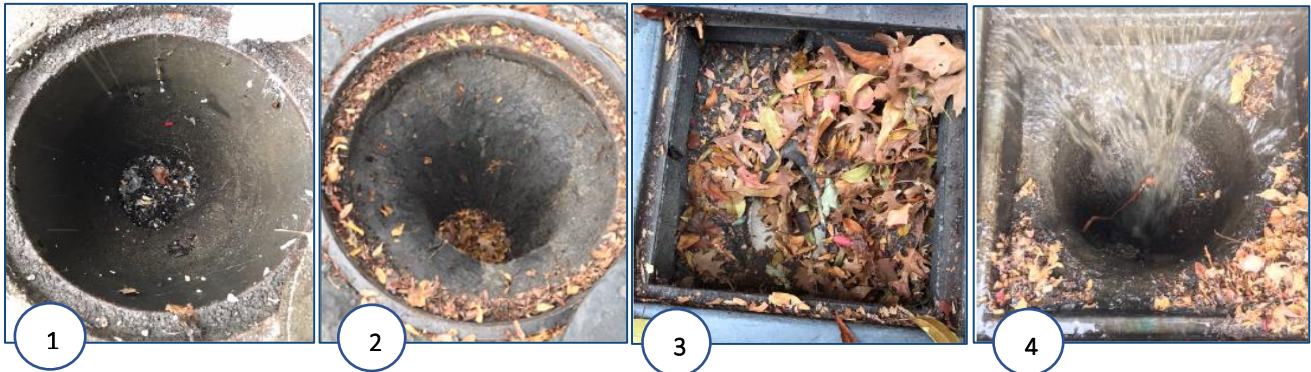
Figure 4.4. (1) Catch basin not wide enough (~15”); (2) Catch basin sump narrows to the outflow pipe; (3) Position of the outflow pipe would block any small FTC device installed; and (4) Catch basin sump not suitable for a device (e.g., square and then rounded or vice versa) (Images courtesy of City of Dublin and SWIMS).
