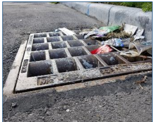
Figure 1.1. Trash accumulating on a storm drain inlet (Photo courtesy of the Santa Clara Valley Urban Runoff Pollution Prevention Program)
