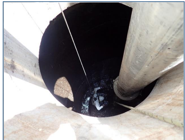
Figure 3.10. Very large HDS unit in San Jose that requires confined space entry to maintain (Image courtesy of City of San Jose staff).
