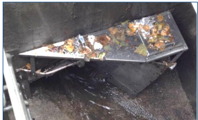
Figure 4.8. Damaged (collapsed) outflow screen type of FTC device (Image courtesy of SCVURPPP and SMCWPPP as included in EOA 2016).
