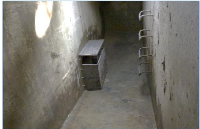
Figure 4.7. Outflow screen installed in a catch basin that requires confined space entry to maintain ( http://unitedstormwater.com/cps.php ).
