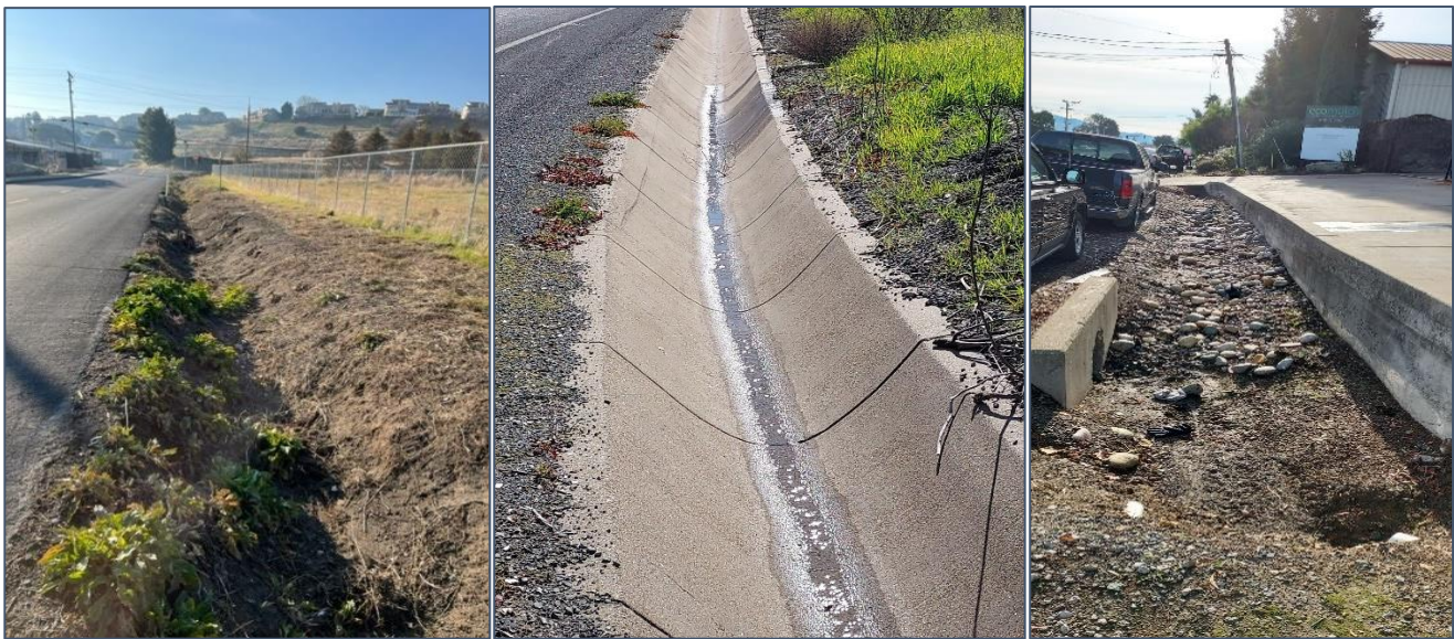
Figure 4.5. Storm drainage infrastructure within the urban limit line in Contra Costa County where installation of Catch-basin types of full trash capture devices is infeasible (Images courtesy of Contra Costa Clean Water Program).
