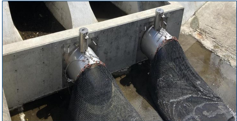
Figure 3.6. NetTech FTC netting system installed in the City of Livermore (Image courtesy of Schaaf and Wheeler Consulting Engineers).
