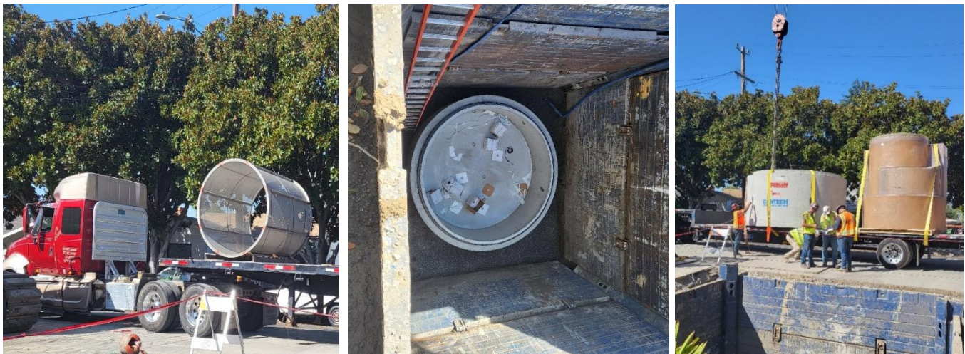
Figure 3.2. Contech CDS® hydrodynamic separator installation in City of Hayward (Image courtesy of EOA, Inc.).
