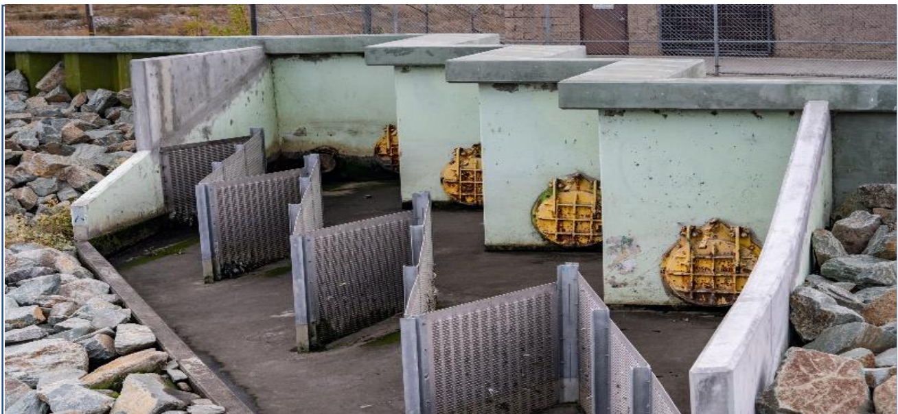
Figure 3.5. Roscoe Moss Gross Solids Removal Device (GSRD) inclined screen configuration installed in the City of East Palo Alto at the outlet of a pump station (Image courtesy of Schaaf and Wheeler Consulting Engineers).
