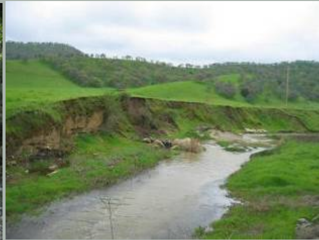
bank erosion: medium
