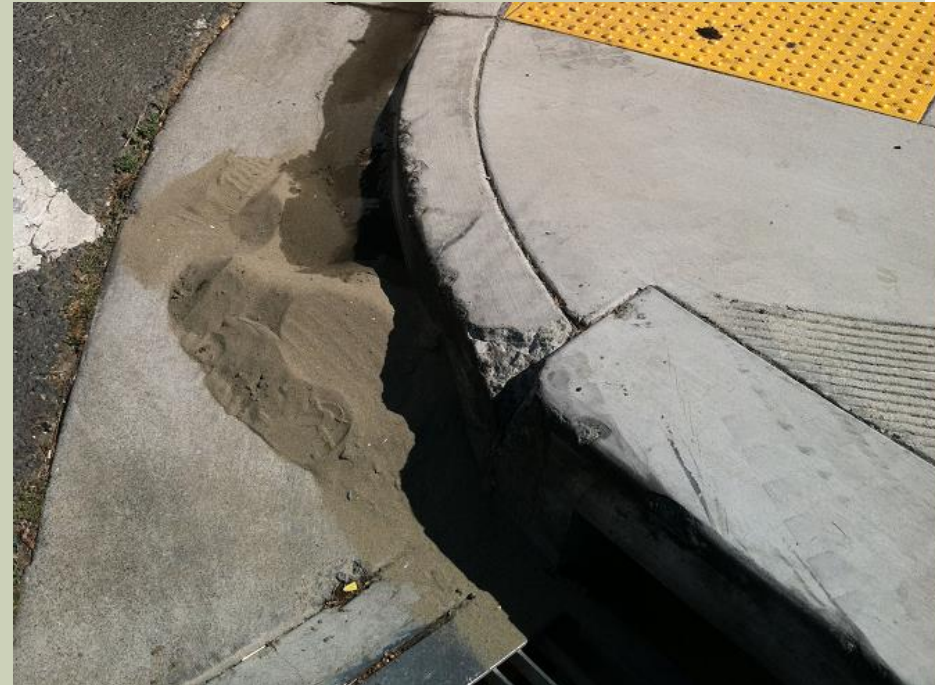
SEWAGE FLOW INTO STORM DRAIN
